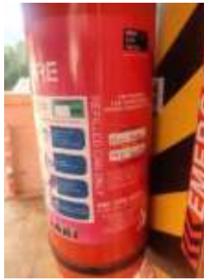
Figure 6. Fire Extinguisher installed
