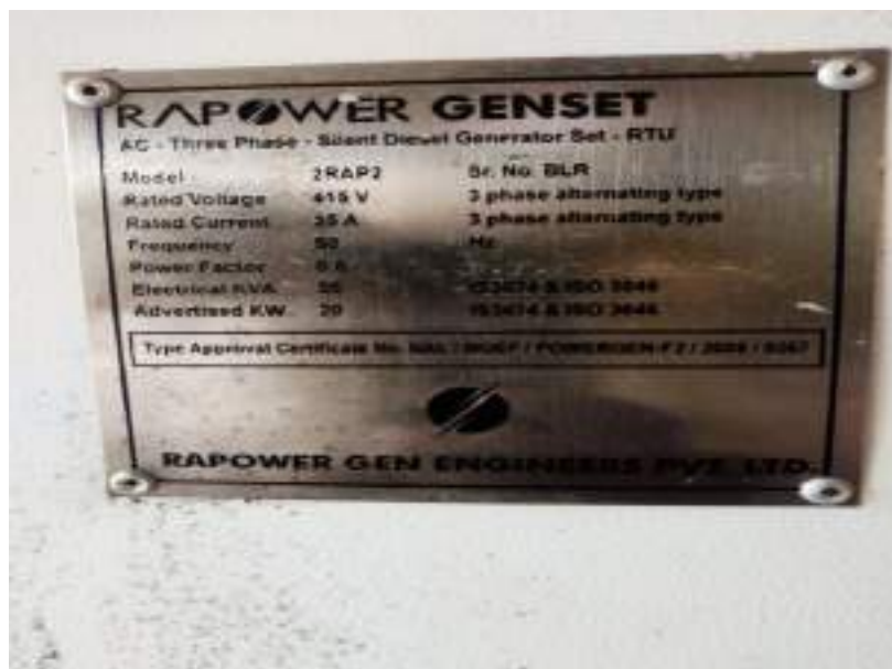
(a) Generator Installed
