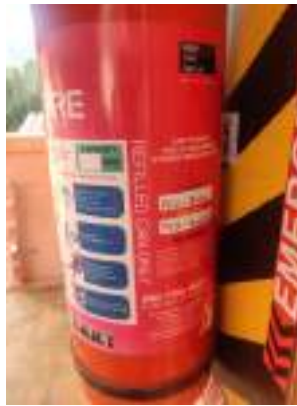
Figure 6. Fire Extinguisher installed
